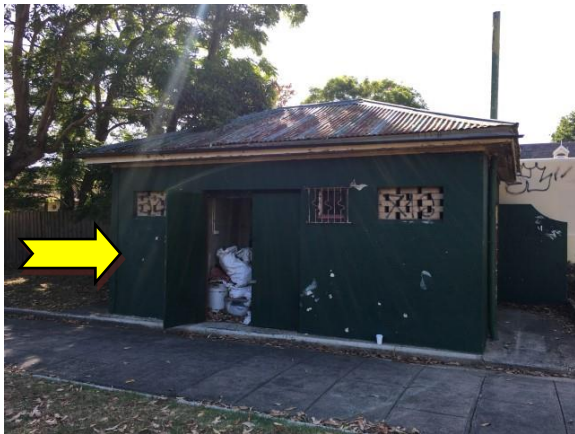
Photo 3. Exterior, throughout, walls – suspected lead-containing green upper coloured paint systems.
