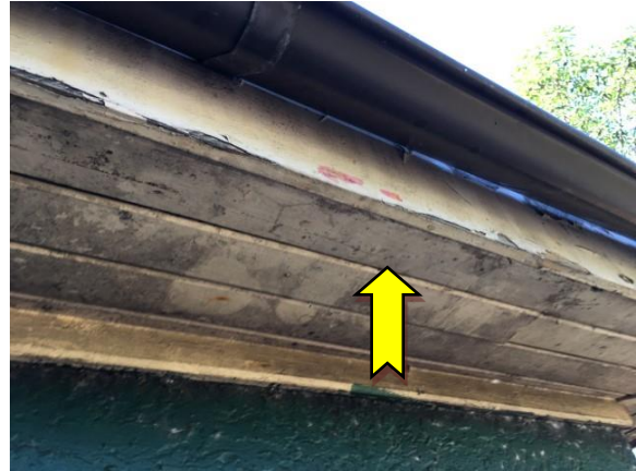
Photo 2. Exterior, throughout, eaves – positive lead-containing cream upper coloured paint systems.
